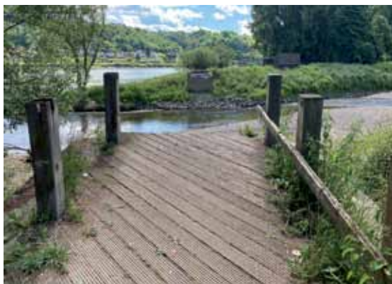
Bicycle bridge over the Ahr had not yet been repaired.
